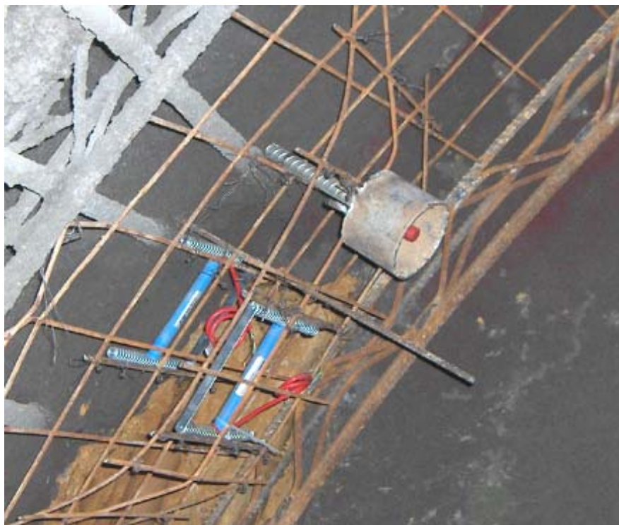
Photo 1 A pair of Encardio-rite model EDS-30V shotcrete strain gages and convergence bolt of an optical target installed before shotcreting of an NATM tunnel.
